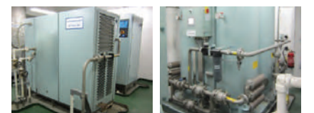
Air Compressor Oxygen Generator
